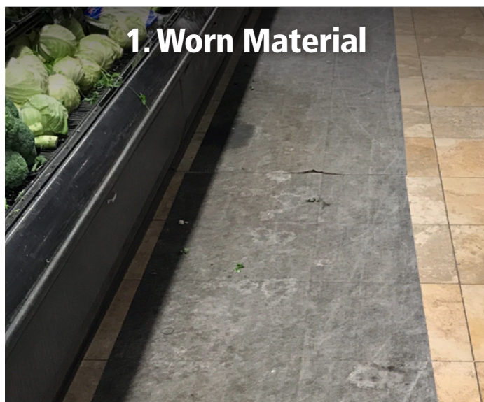
Lifting seams, frayed edges, overall worn and stained appearance: REPLACE.
