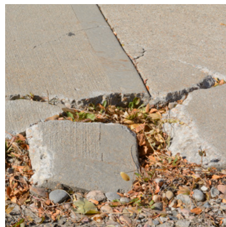
Cracked and crumbling sidewalks make walking dangerous for employees and visitors.
