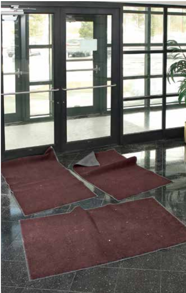
Fragmented mat coverage becomes an obstacle course of tripping hazards.
